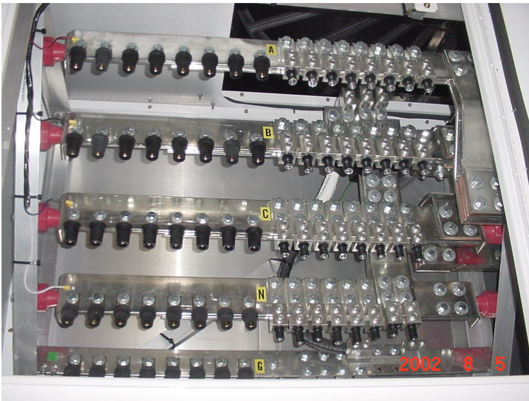
Photo 8: Cable Terminals for a Cummins Portable 2000KW, 480V Unit (All Connections are sized for 4/0 Cu Conductors)
