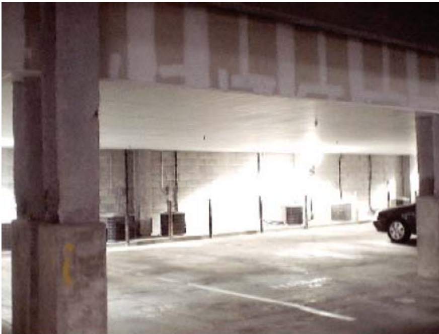
Photograph No. 2 - Garage Plenum where electric heaters are installed to prevent freezing of fire sprinkler system in the garage.
