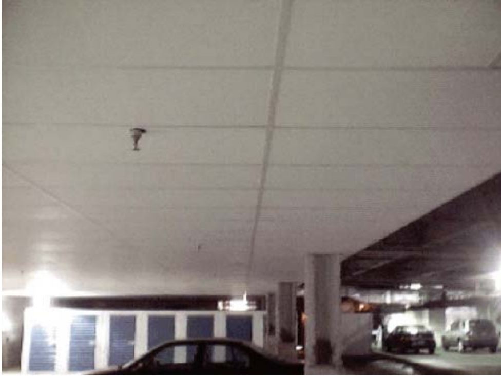
Photograph No. 1 - Fire sprinkler heads in the garage.
