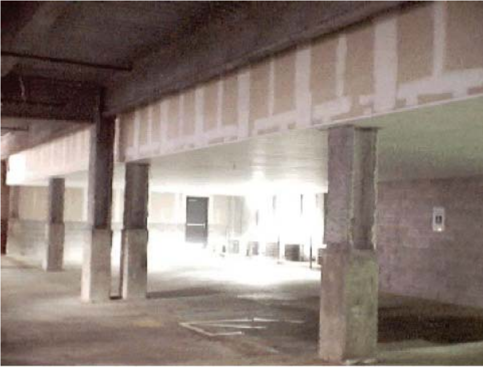
Photograph No. 3 - Garage Plenum where electric heaters are installed to prevent freezing of fire sprinkler system in the garage.
